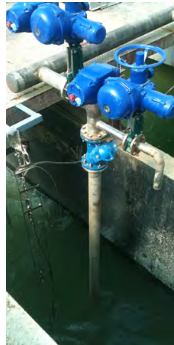
The waste water treatment Adler
